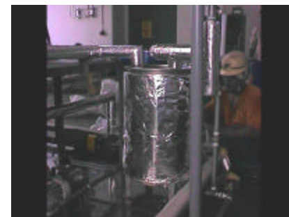
Cooling/Heated Water circulation Tank=>
