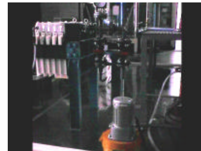
Progressive Cavity Pump & Filter Press =>
